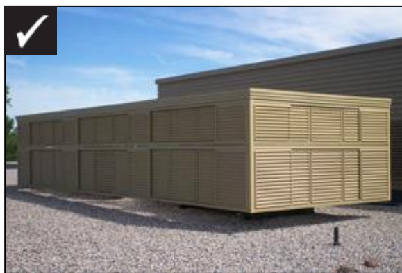
Screened roof-top equipment
