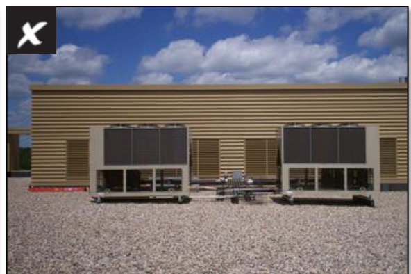
Unscreened roof-top equipment
