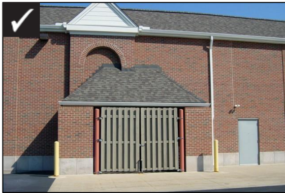
Screened ground-level equipment
