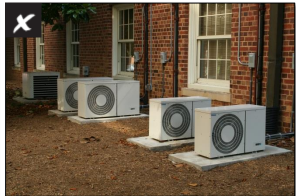
Unscreened ground-level equipment
